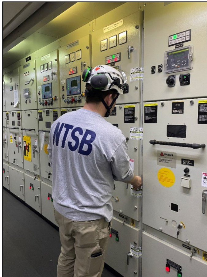
Figure 8. An NTSB investigator examining the Dali 's HV switchboard (which houses the HV bus) and applying tamper-evident preservation seals.
